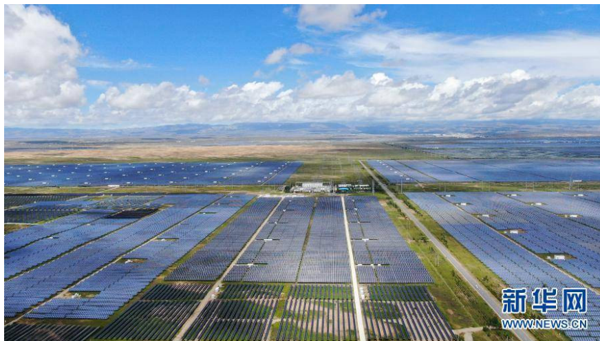
Picture 2 Photovoltaic power station in Talatan Green Industry Development Park, Judi County, Hainan Tibetan Autonomous Prefecture, Qinghai Province
