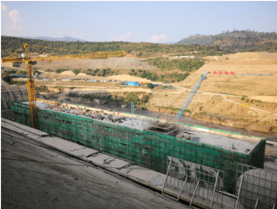
Picture 1 The switching station of the Karot Hydropower project in Pakistan was successfully capped in June 2020
