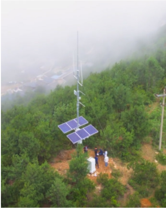
Picture 6 Huawei's RuralStar in the Liangshan region
